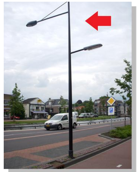
Figure 8 Innovative lighting simultaneously provides light for streets and cycle tracks.
